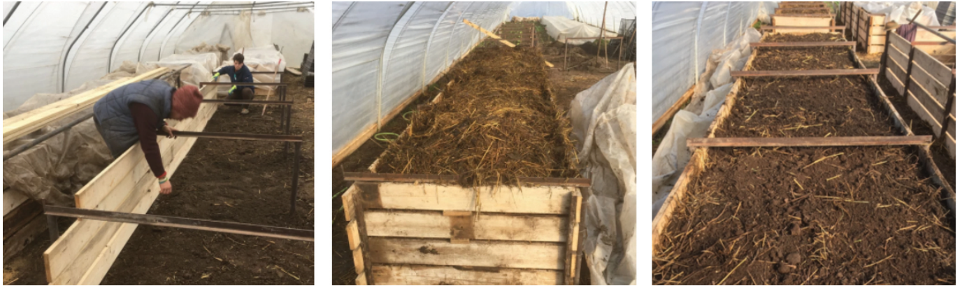
Figure 4.44: Constructing a frame for a manure heated germination bed, hotbed filled with manure. Credit: Zsámboki Biokert
